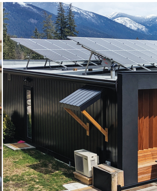
7.7 kW rooftop solar photovoltaic array connected to a grid tie-in for net metering.
