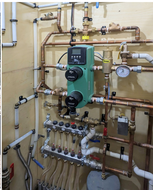
In-floor radiant heating and cooling system, supplied by the AWHP, utilizing the inherent thermal mass of the building.
