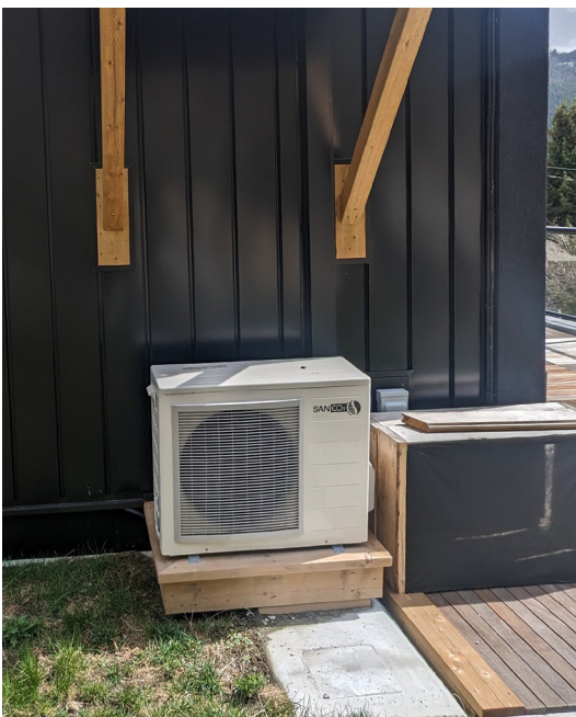
Air-to-Water heat pump (AWHP) outdoor unit providing heating and cooling to the building.
