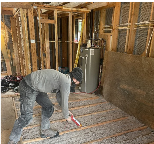
Insulating the floor with cellulose to reduce heat loss, while also using a low embodied-carbon material.
