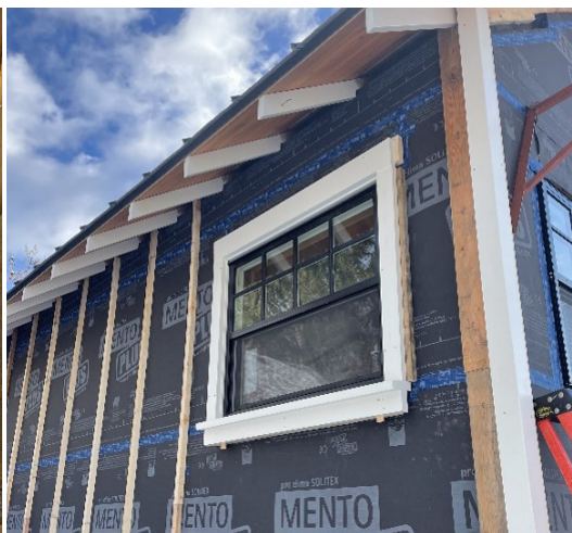
Window detail with rainscreen membrane to mitigate impacts of air leakage in wall penetrations.
