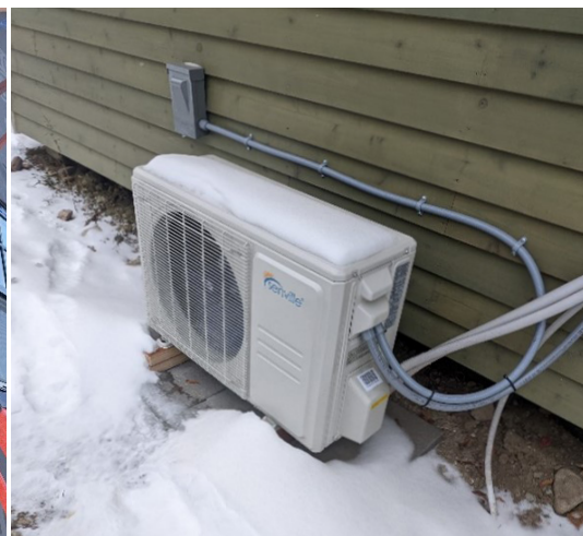
Air-Source heat pump providing heating and cooling via an exterior fan coil unit.
