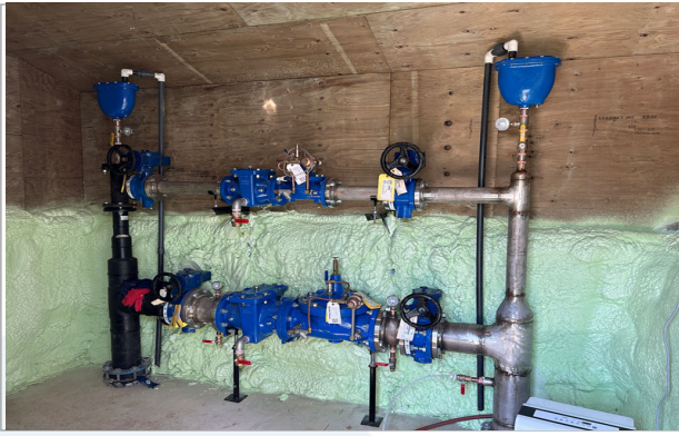
New Pressure Reducing Valve Station
