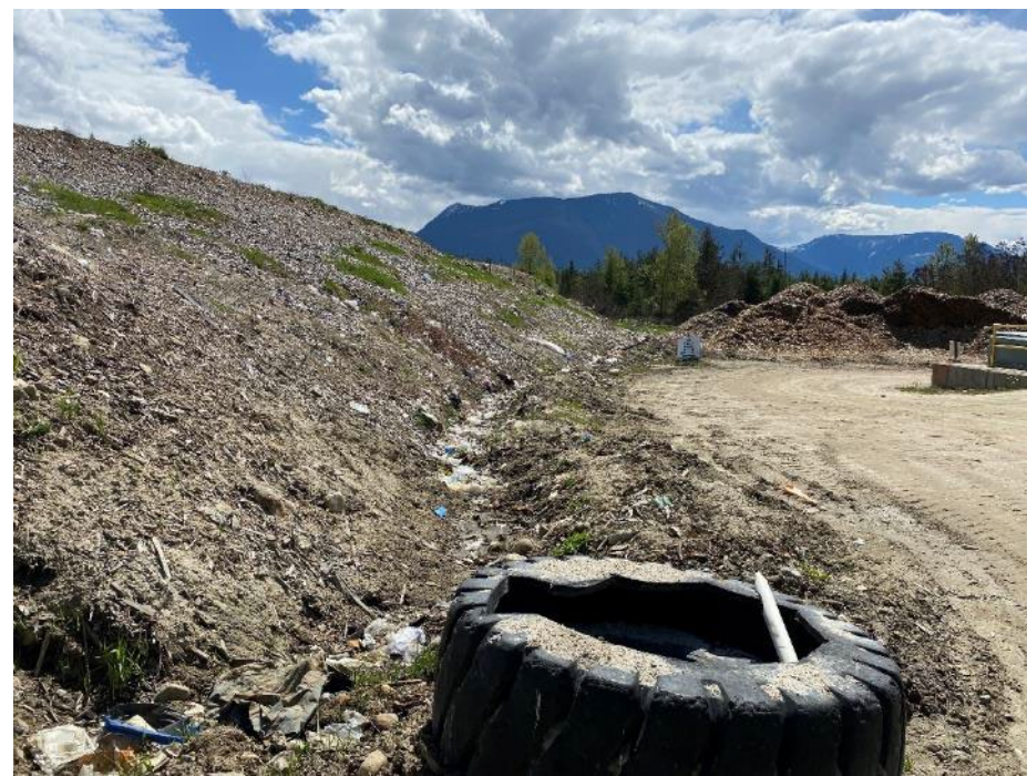
Photo 16: Drainage ditch running between Main pile and wood pile with standing water present (May 3, 2024)
