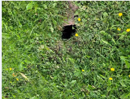
Hole in Exposed Steel Pipe
