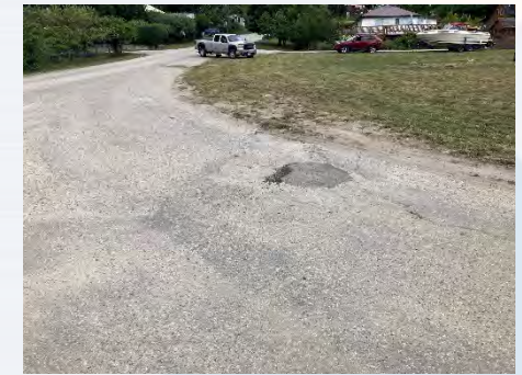
No Catch Basin at Tee
