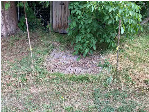
Wood Catch Basin Cover
