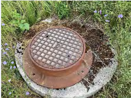
Unsecured Cover – No Grate
