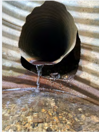
Pipe Miss Aligned
