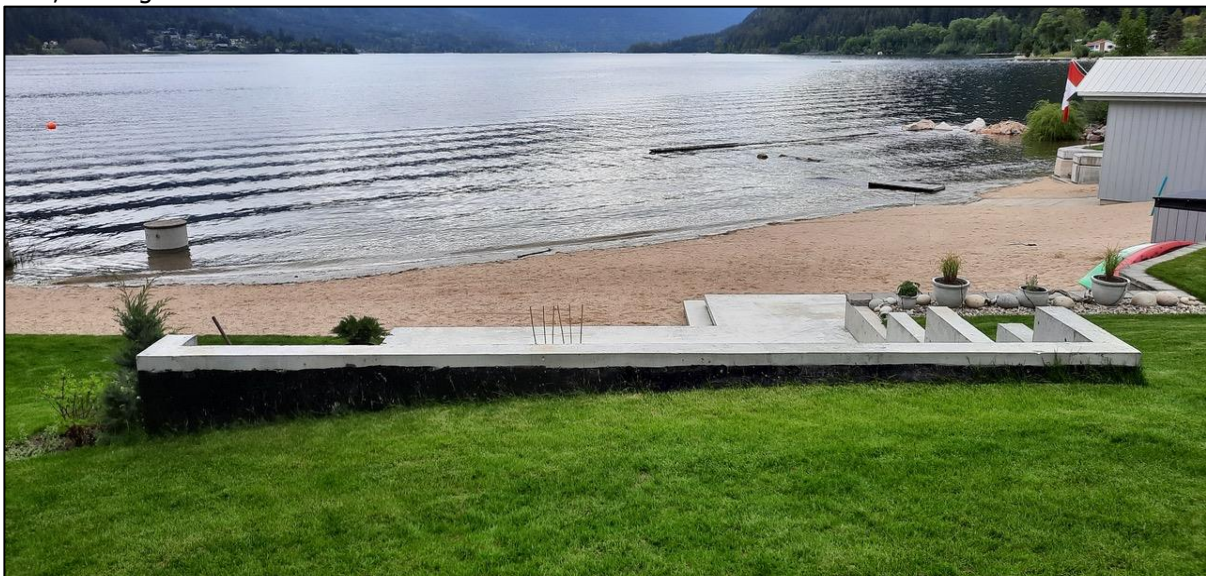
Photo 2. Concrete foundation for the proposed boathouse and landscaping in relation to the foreshore, looking north.
