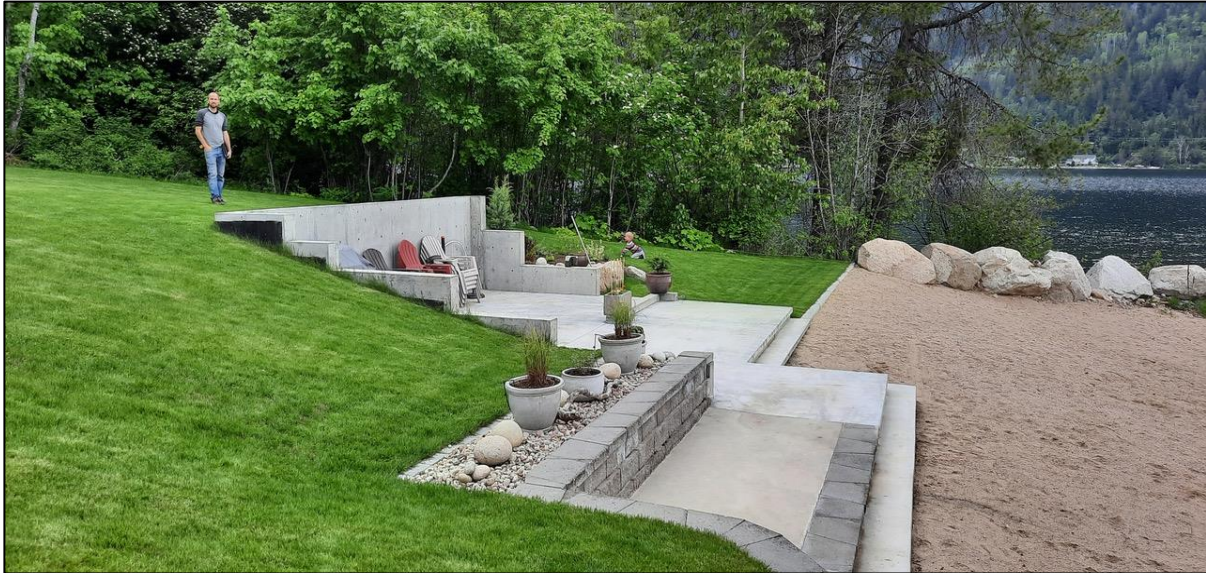
Photo 1. Concrete slab for patio and proposed boathouse, and landscaping partially within the 15 m WDP area, looking west.
