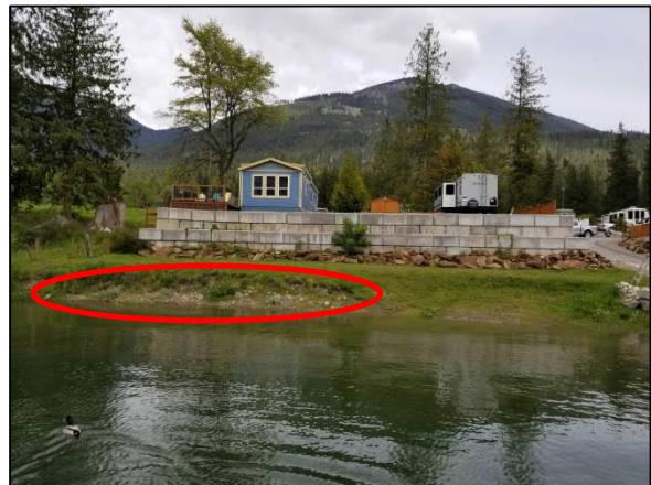
Photo 11. View of foreshore and visible erosion fronting western retaining wall, looking north, May 31, 2022.
