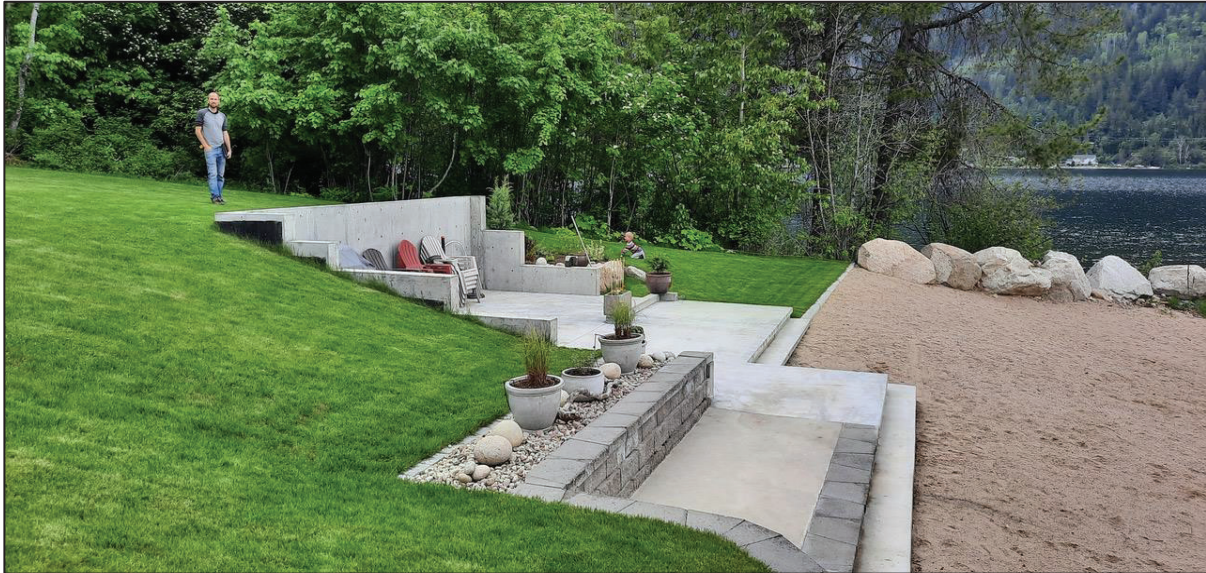
Photo 1. Concrete foundation for the proposed boathouse and landscaping within the 15 m WDP area, looking west.
