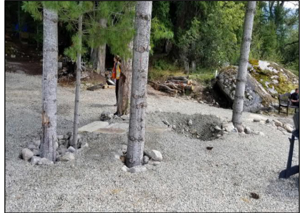
Photo 14. Backfill placed around conifer trees in front of existing cabin at north portion of property.
