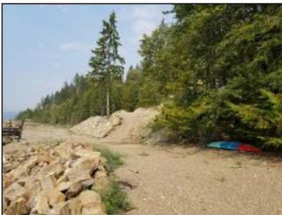
Photo 11. View of backfill and rock placed around mature fir tree along foreshore.
