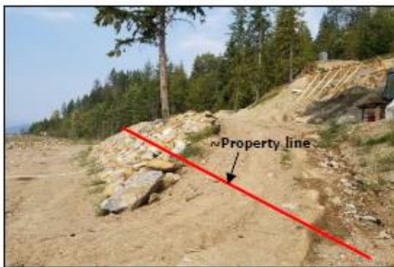
Photo 3. Fill encroachment along the foreshore, looking north, Sept 8, 2021.
