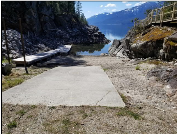
Photo 7. View of concrete boat ramp and floating dock at boat launch area.
