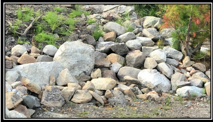
Photo 6: Rip rap area to be removed and planting of conifer and deciduous stems to be undertaken
