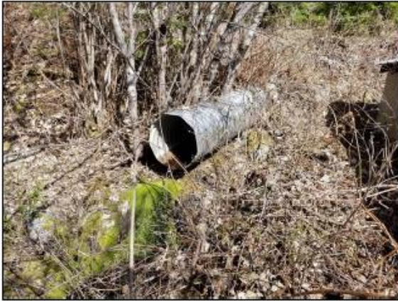
Photo 13. Perched culvert outlet downstream of Fortis easement proposed Lot B.
