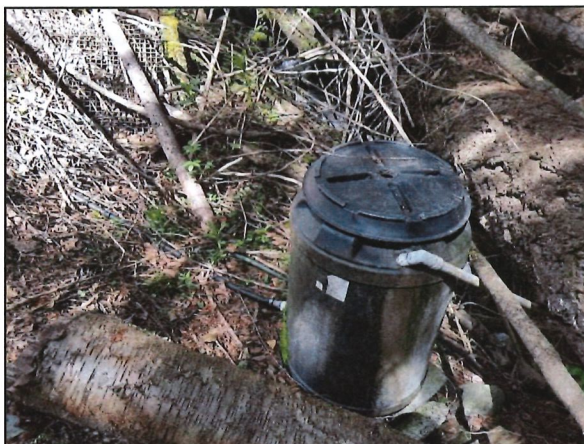
Photo 12. Water intake near lower end of creek.
