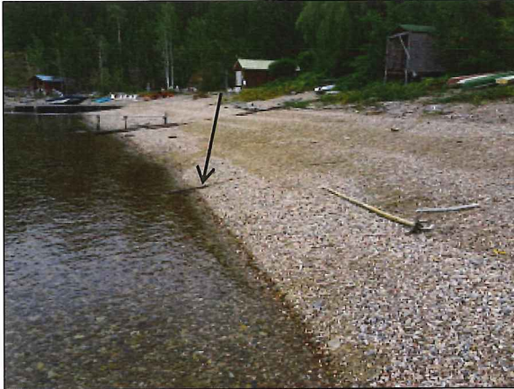
Photo 7. Water intake line for Lot 2.
