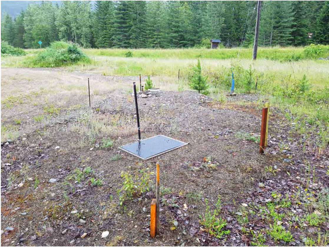
Figure 7: Existing Servicing Installed for all Proposed Lots
