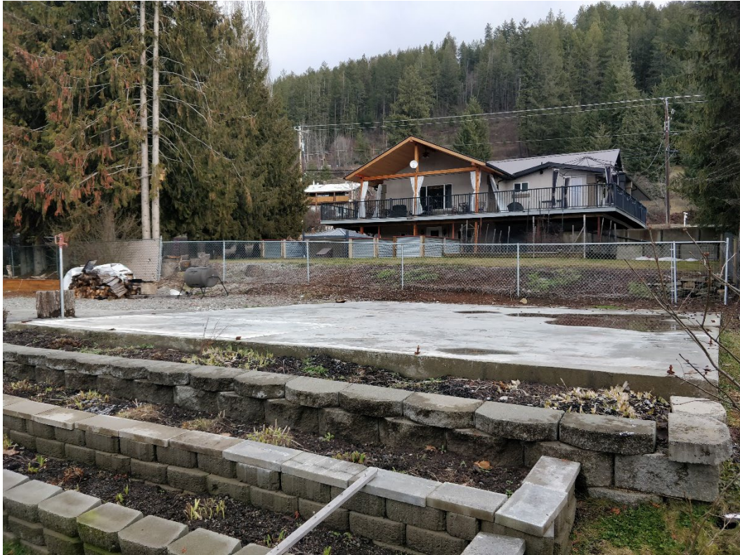
Figure 6 – View looking east towards the existing concrete slab that remains from the original building that burnt down.
