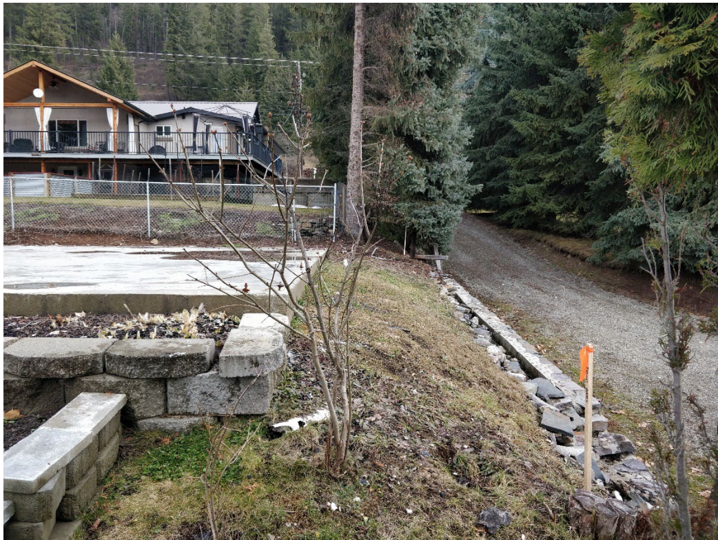
Figure 7 – View looking east that shows the 1.5 metre distance from the existing concrete slab to the property line.
