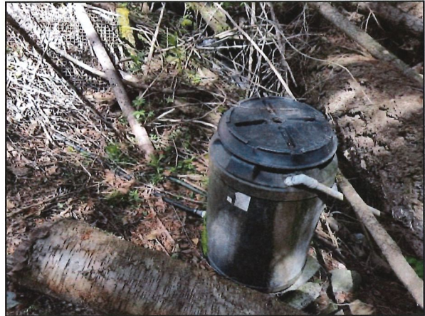
Photo 12. Water intake near lower end of creek.
