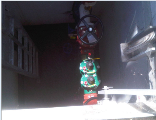
Vault from City of Castlegar supply housing meter and back-flow assembly
