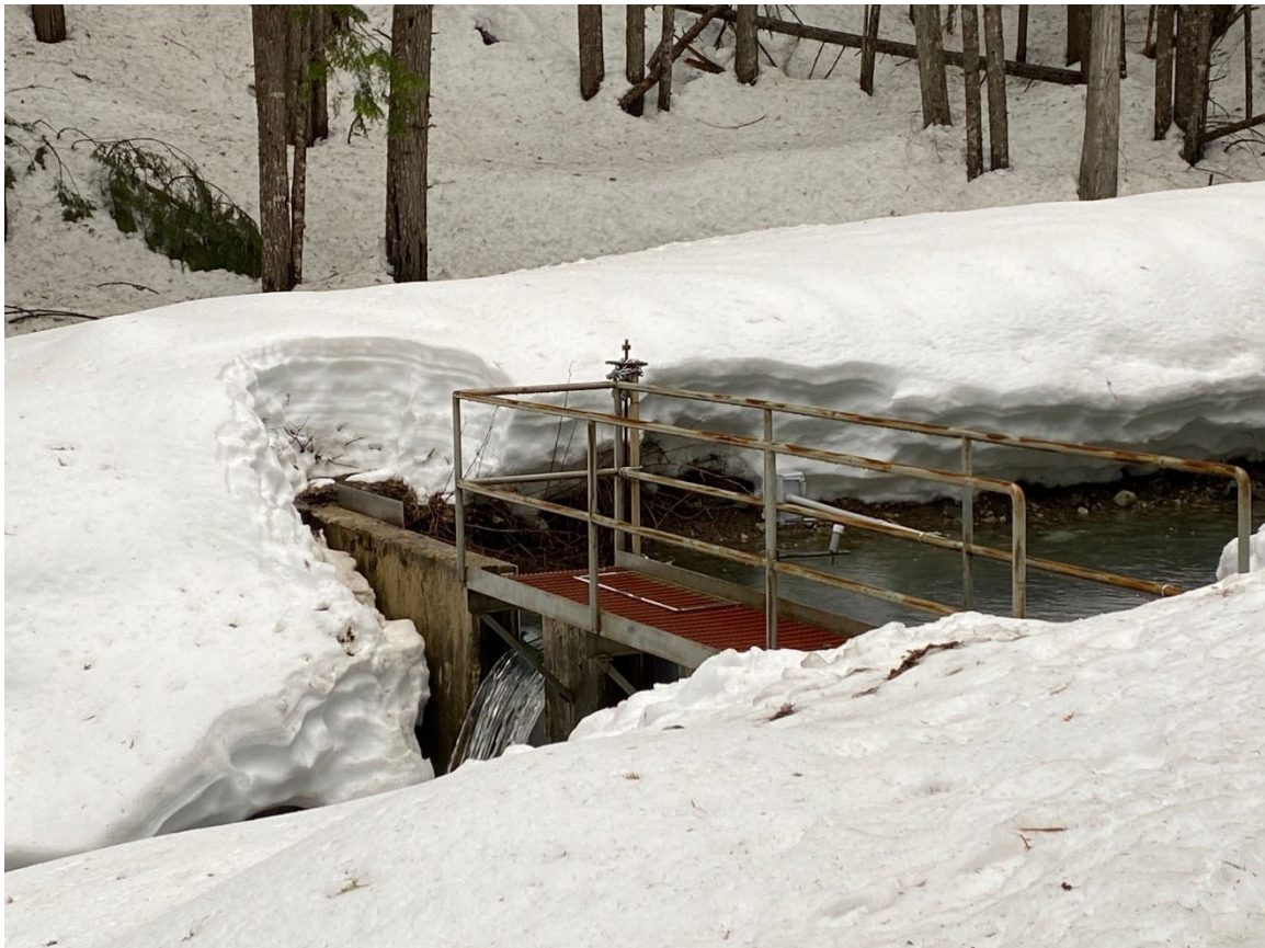
Quartz Creek Flow Weir Discharge – 31 March 2020
