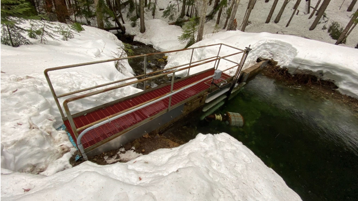
Quartz Creek Ymir Water Intake – 31 March 2020
