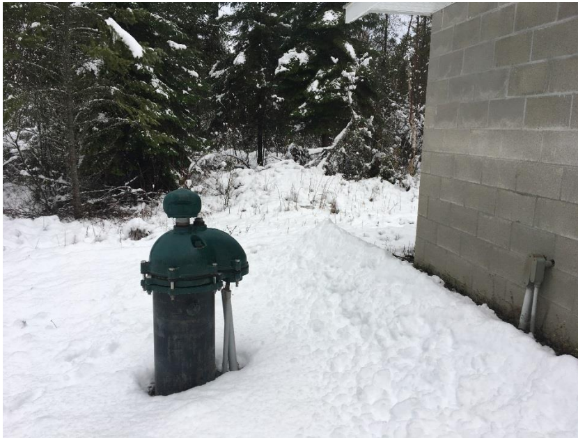
Figure 3: 250mm Diameter Production Well
