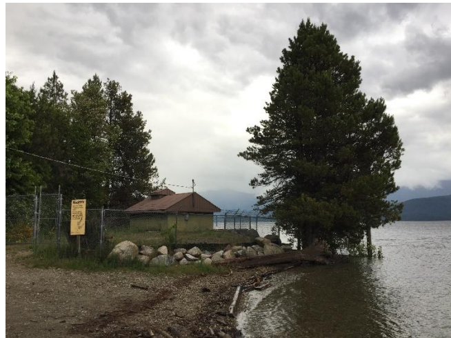
Balfour Water, Kootenay Lake Pump Station
