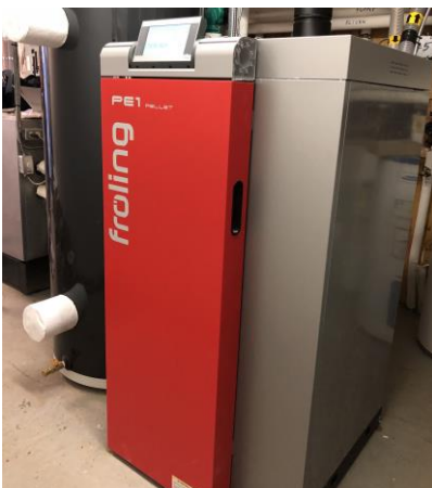
Figure 16. Fröling PE1 Wood Pellet Boiler (20 kW th )
