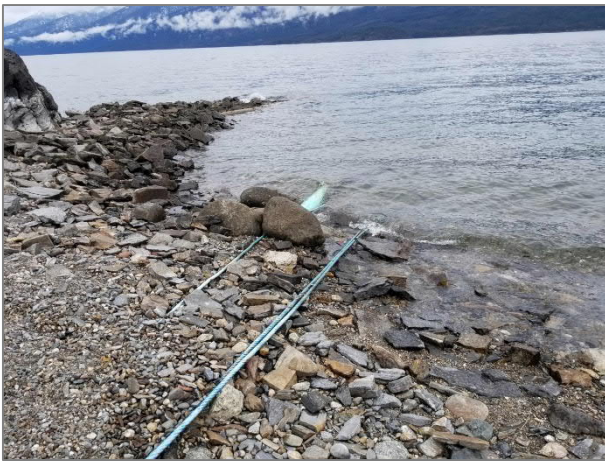
Photo 5. View of existing WWTP discharge line entering Kootenay Lake.
