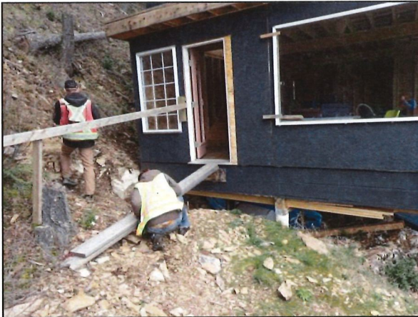
Photo 7. Approximate location of proposed deck off south door of cabin to connect existing staircase down to foreshore area, April 14, 2017.
