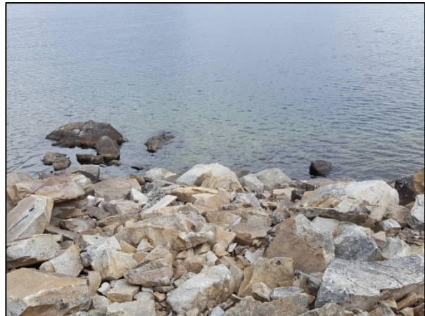
Photo 13. View of boulder and cobble substrate material overlying bedrock in front of Lot 1.
