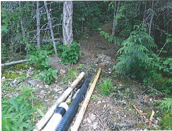
Photo 7. Water intake line through riparian area
