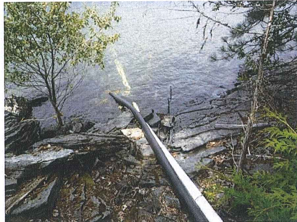
Photo 8. Water intake line at foreshore.
