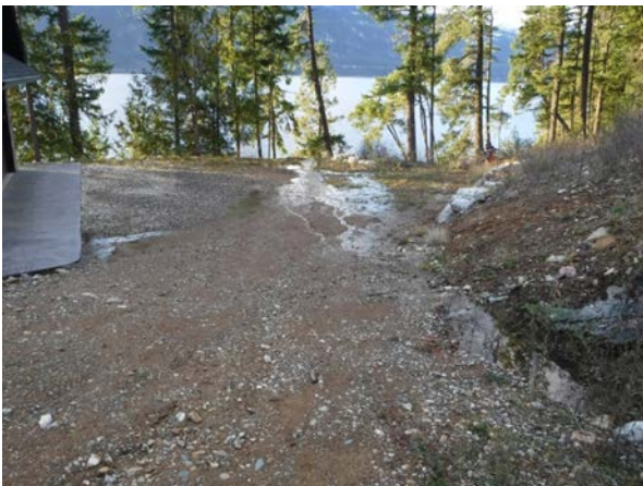
Photo 9. View of surface drainage issues on Lot 9, Phase 1.
