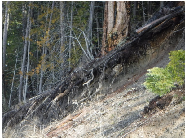
Photo 8. View of undercut bank and exposed tree roots at top of bank.
