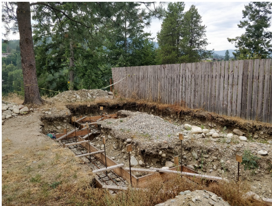
Figure 5: Facing North West toward the building site. The wooden fence is the approximate location of the northern interior lot line.
