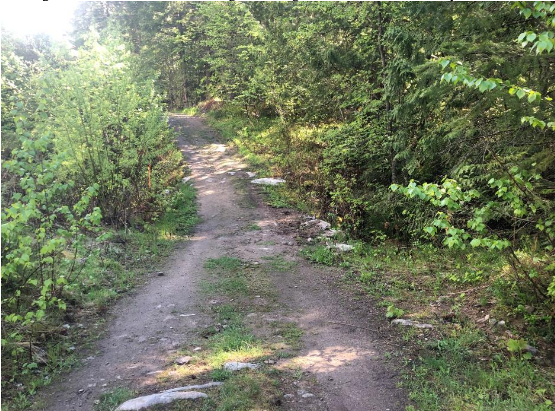
Photo 13: Road crossing at powerline looking north. Flow left to right threw 900 mm CMP. May 11, 2021
