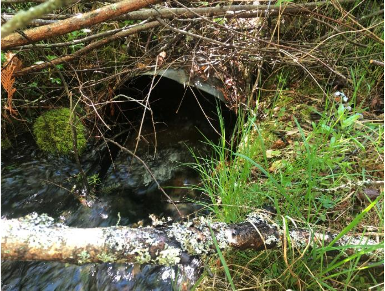
Photo 5: View of entrance to 600 mm diameter culvert at Annable Rd crossing at on north end of the property approximately 60 m upstream from dwelling. May 11, 2021
