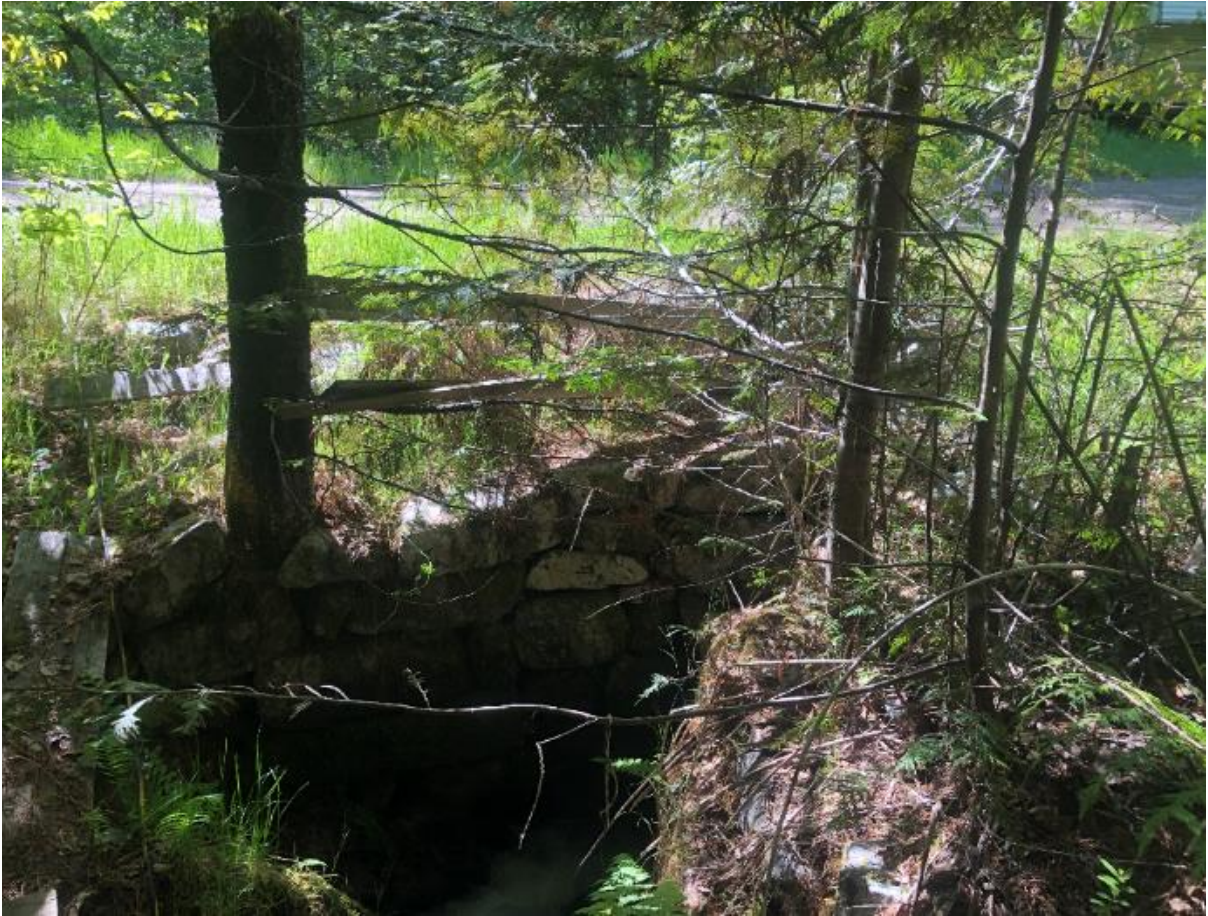
Photo 7: View at entrance to 600 mm diameter culvert crossing at private road crossing approximately 340 m upstream from the Annable Road crossing. Channel gradient 10% May 14, 2021
