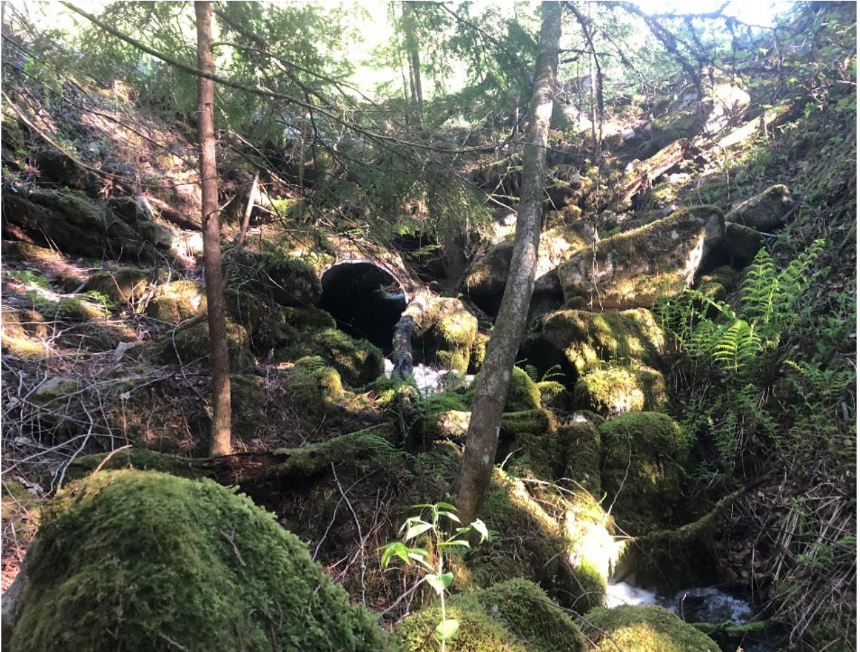
Photo 14 : View looking upstream at downstream side of 900 mm CMP road crossing at powerline. May 14, 2021
