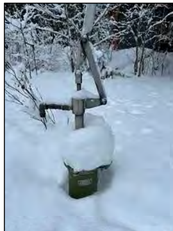
Photo 18. View of water pump at well location.
