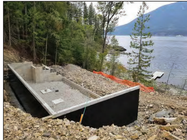
Photo 4. Current view of new house foundation and elevated bench along west side of house, Sept 22, 2022.
