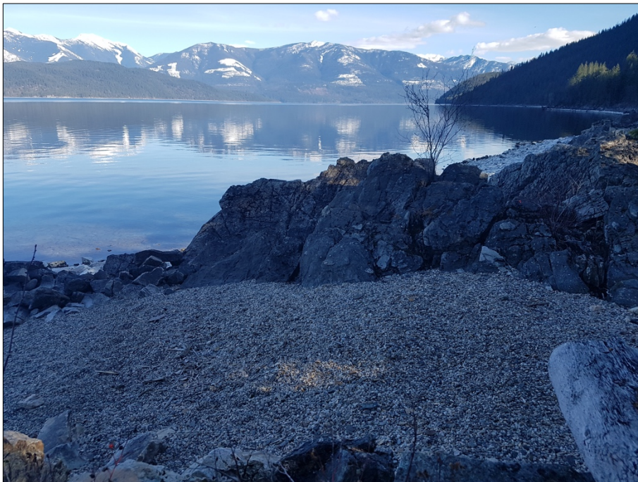
Photo 2. View southeast of the foreshore of the lot. Note the foreground where geotextile has been overlaid with imported pea gravel to improve access to the naturally rocky shoreline.
