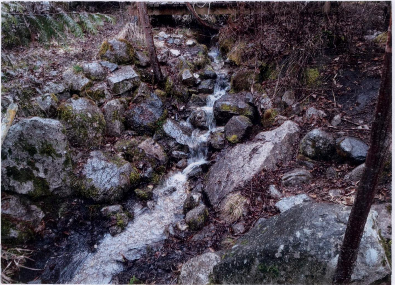
Photograph: Crystal Creek above Annable Rd Culvert at 12 gallons per minute flow.
