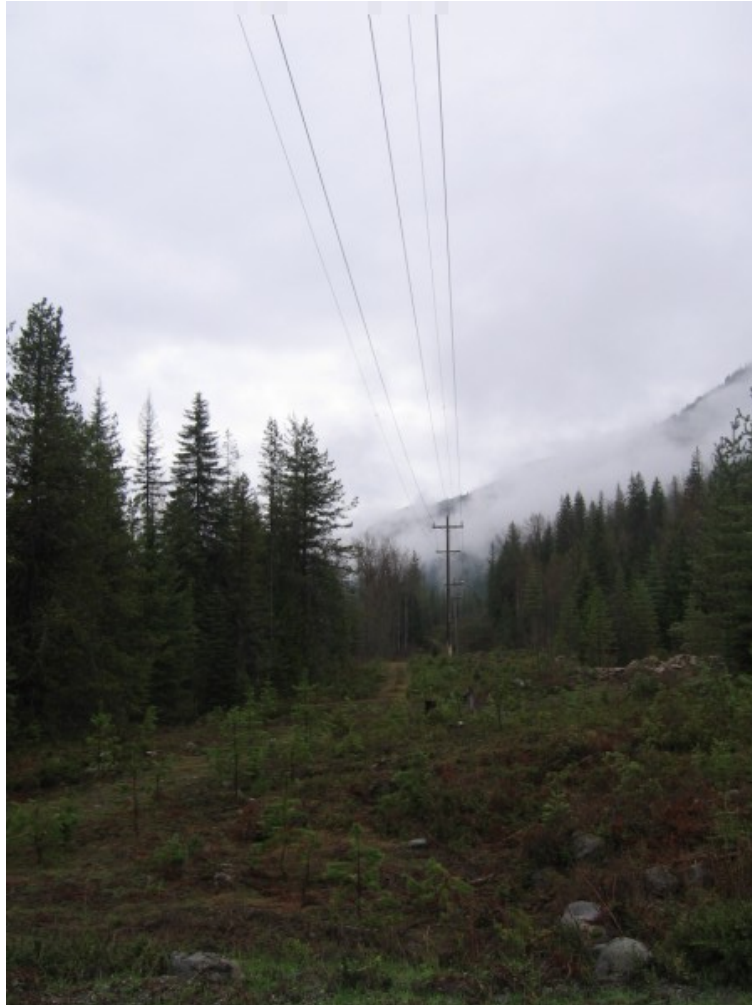
Figure 3. Wood pole transmission infrastructure.
