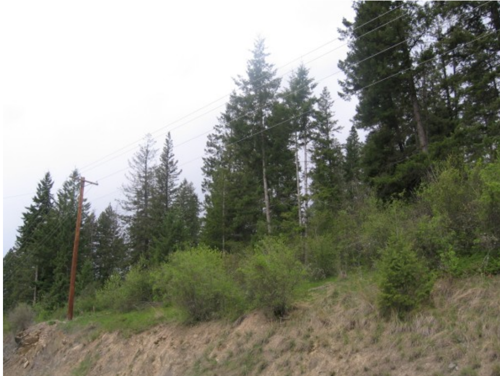
Figure 3. Wood pole distribution infrastructure.
