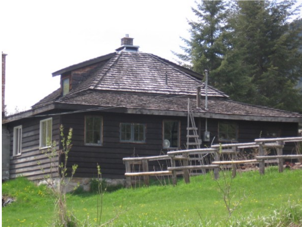
Figure 3. Photograph showing unrated roofing material and wood siding on a house in the Winlaw Fire Protection Area.
