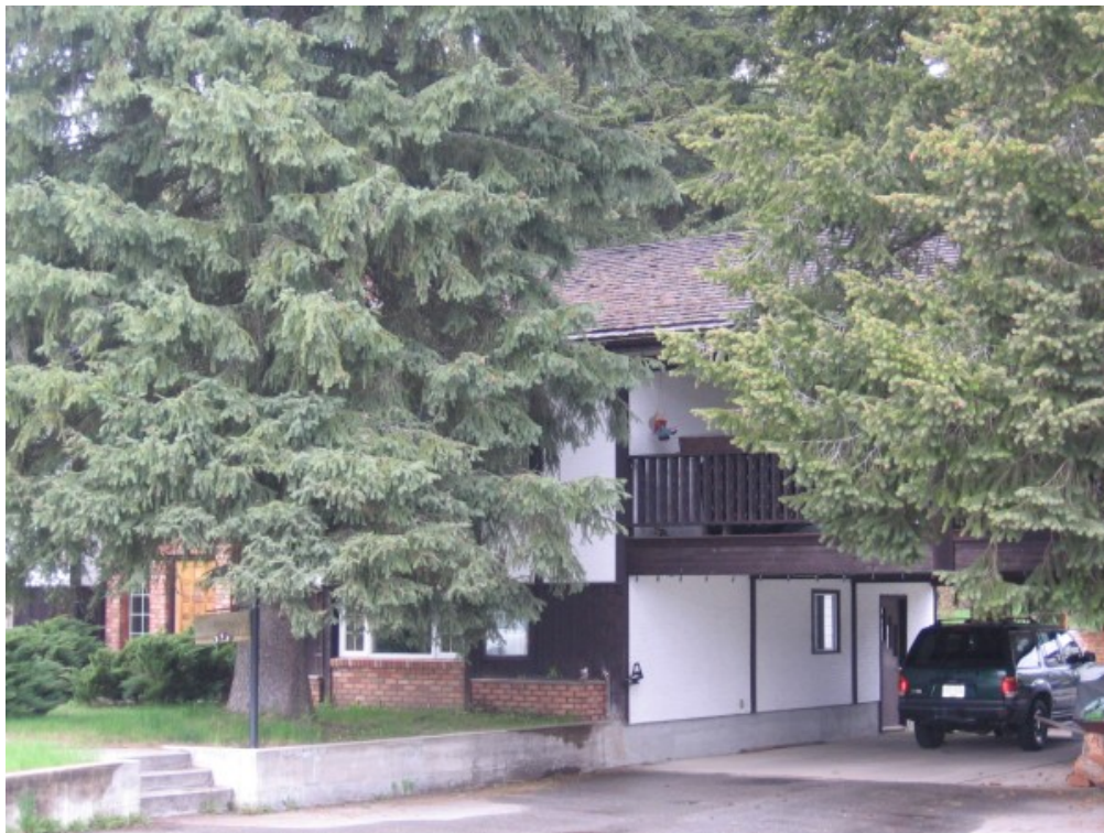
Figure 3. Example of home with wood siding and no setback to vegetation.
