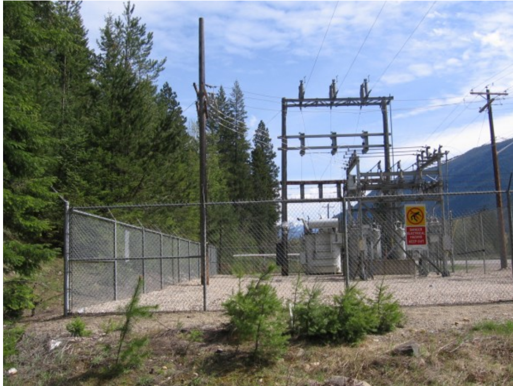
Figure 3. Transmission infrastructure in Passmore.
