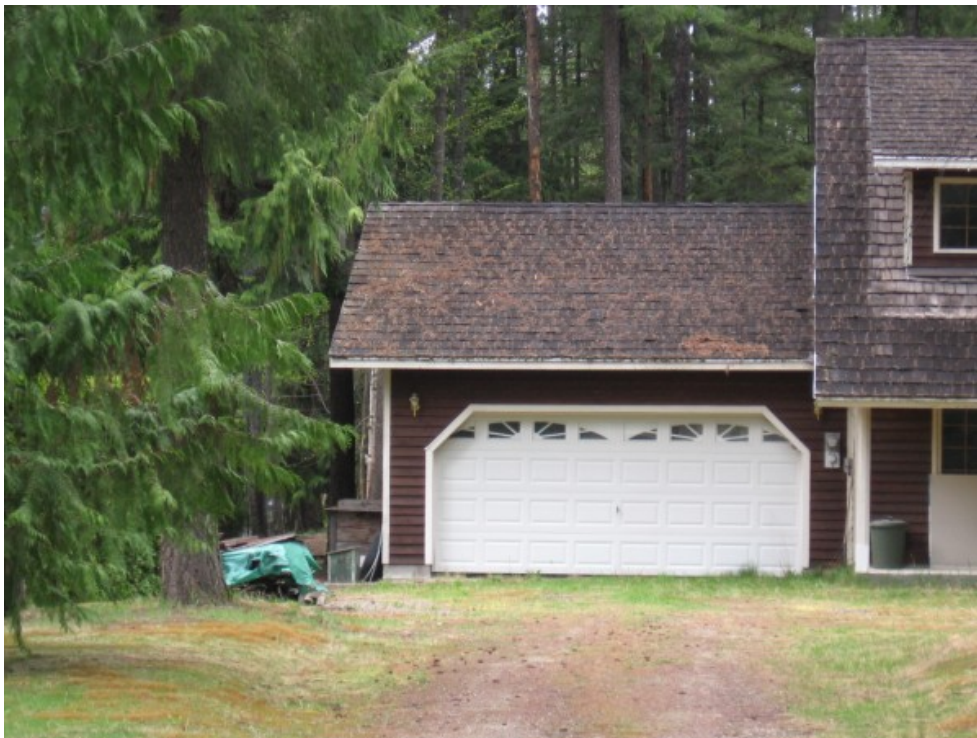
Figure 3. Photograph showing unrated roofing material present on many homes within the wildland urban interface.
