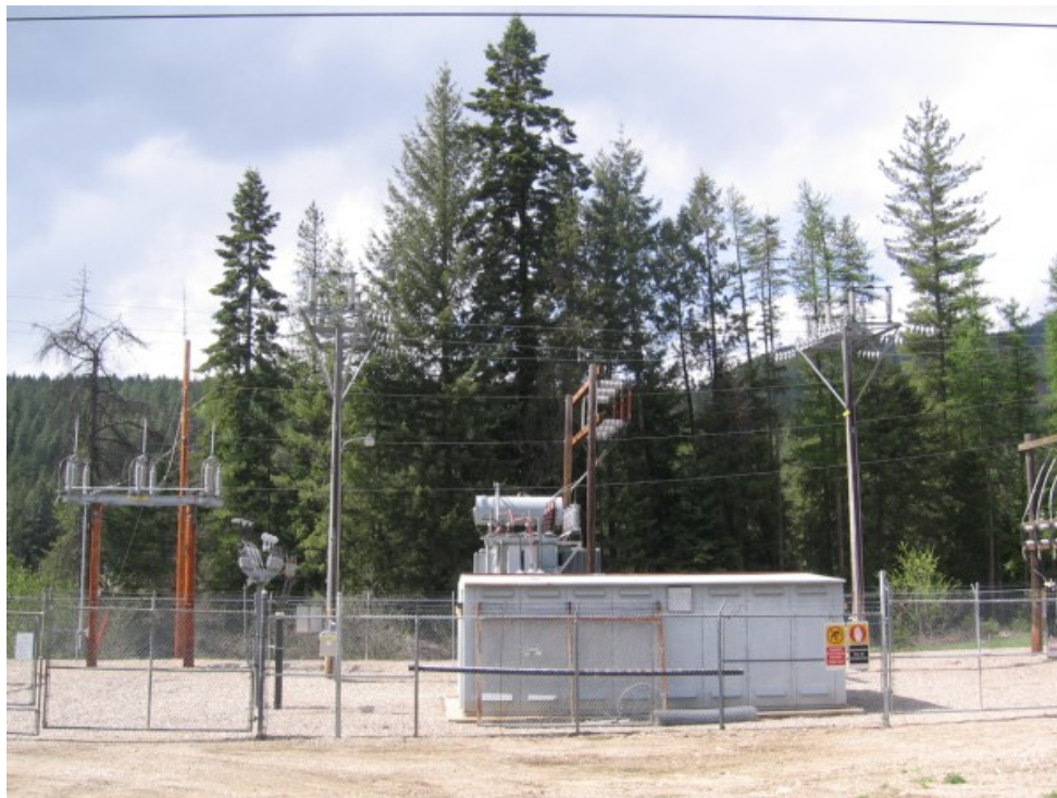
Figure 3. Electricity distribution infrastructure in Crescent Valley.
