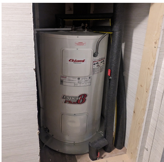
Electric water heater provides hot water for the home using a low GHG emission energy source.
