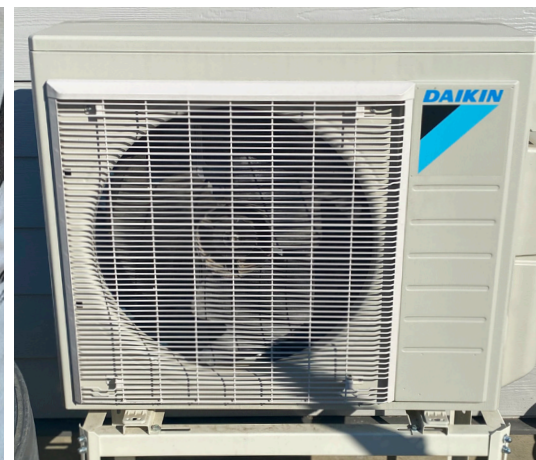
Daikin Air-Source heat pump providing heating and cooling via four interior fan coil units.
