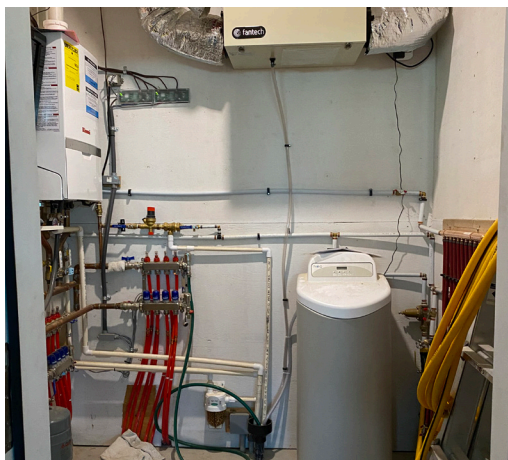
Mechanical room showing underfloor heating piping, HRV unit and backup gas boiler.
