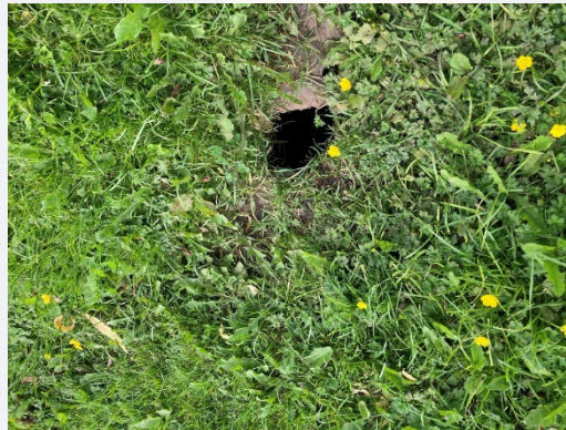
Hole in Exposed Steel Pipe
