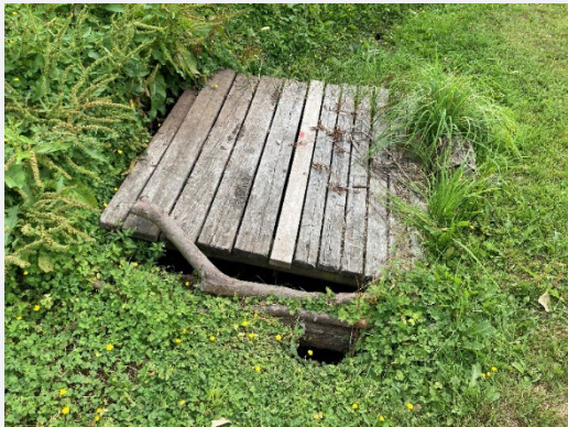
Wood Decking Catch Basin Cover Safety Concern for Traffic and Pedestrians
