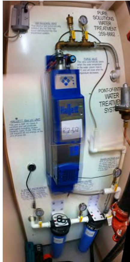
Figure 9: Point of Entry Treatment System
