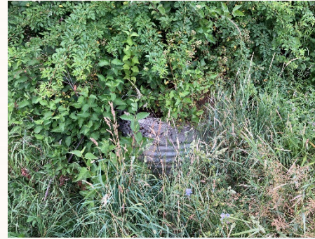
Surface Water Cannot Flow In
