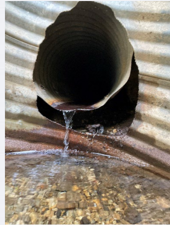
Pipe Miss Aligned
