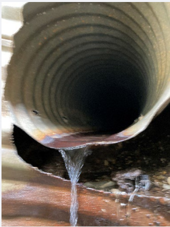
Pipe Not Grouted
