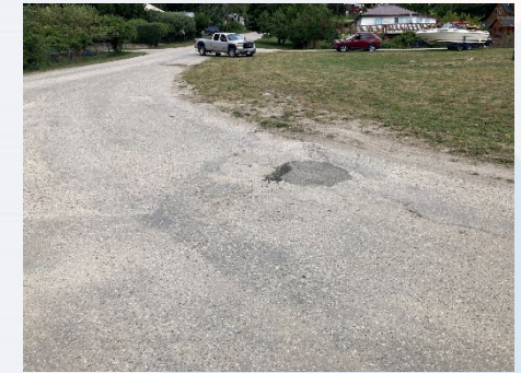
No Catch Basin at Tee
