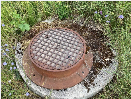
Unsecured Cover – No Grate
