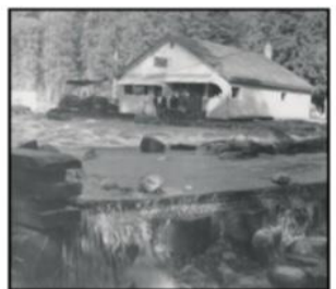
Flood damage to building and highway bridge, 1956 (Fred and Audrey Heddle Collection)
