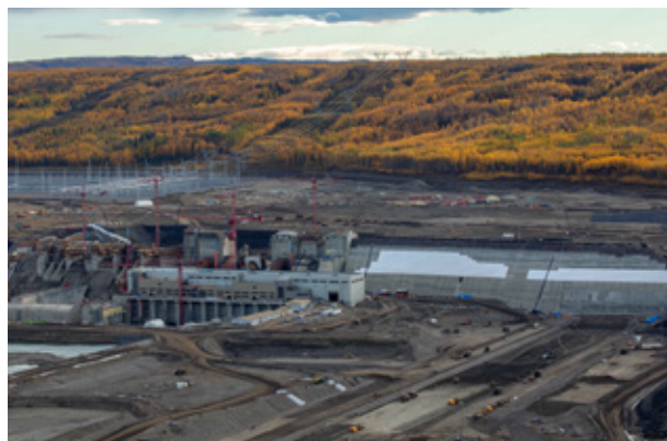
A view of the Site C dam core trench, dam buttress, powerhouse, spillways, and the operational substation in the background.
