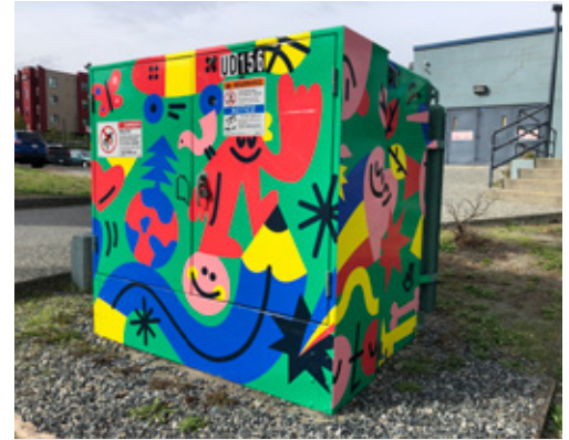
Example of a decorative wrap on our pad-mounted equipment.
