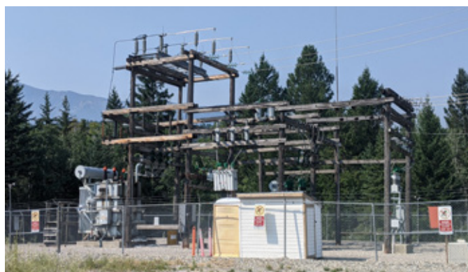
Equipment at Canal Flats Substation (pictured) and on poles throughout the community will be replaced between fall 2021 and fall 2022 to improve reliability to our customers in the southern Columbia Valley.
