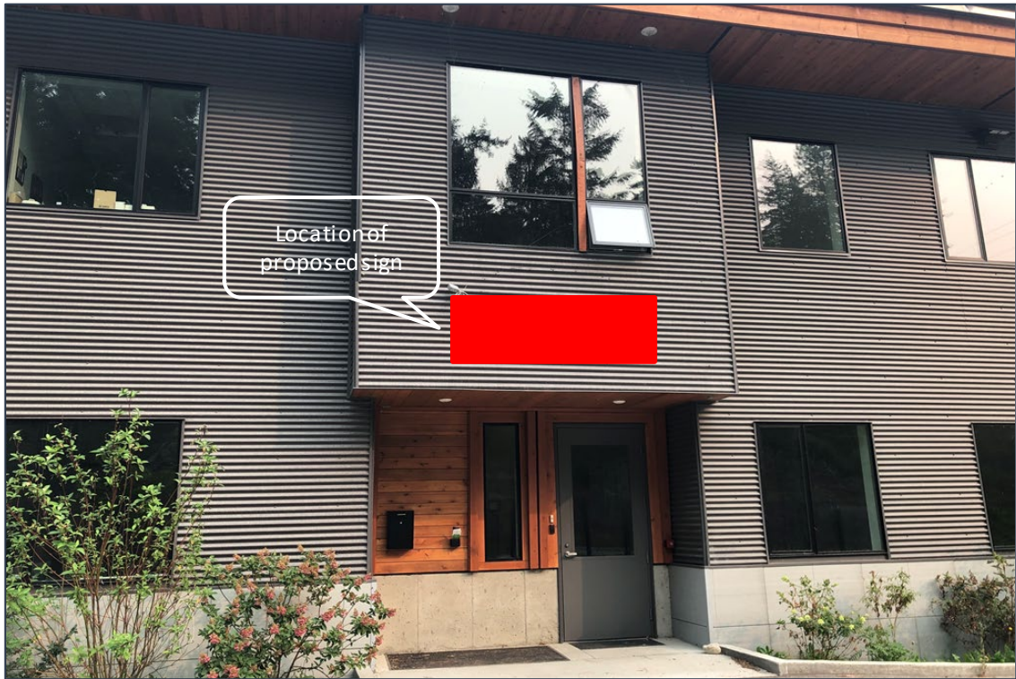
Figure 3: Front entrance of subject building, where the illuminated sign is proposed to be located
