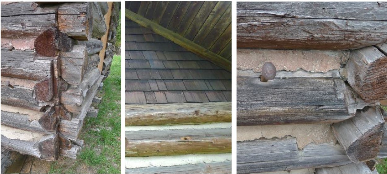
Top: showing side elevation and large opening created when the cabin was adapted as a warming hut for the proposed ski hill, this replaced a small window opening
