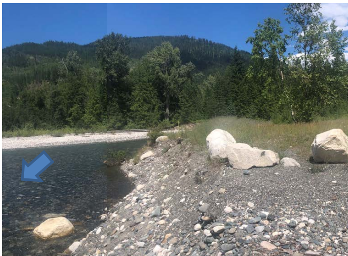
Photo 21. Standing at the Wilson Creek outlet on Slokan Lake on the left bank looking upstream at bank erosion. Photo: BGC, July 26, 2019.
