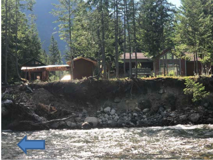
Photo 13. Standing on the left bank of Wilson Creek looking across at bank erosion on the right bank just downstream of the Hwy 6 bridge. Photo: BGC, July 26, 2019.
