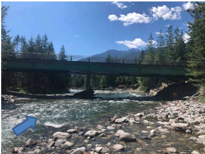
Photo 11. Standing on the right bank of Wilson Creek looking downstream at the Hwy 6 bridge. Photo: BGC, July 26, 2019.
