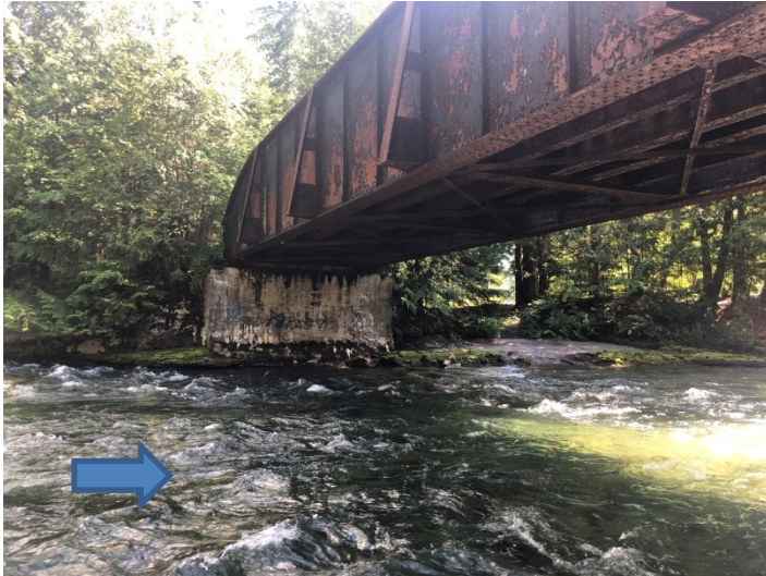
Photo 16. Standing on the right bank of Wilson Creek looking across at the left bank and the railway bridge. Photo: BGC, July 26, 2019.
